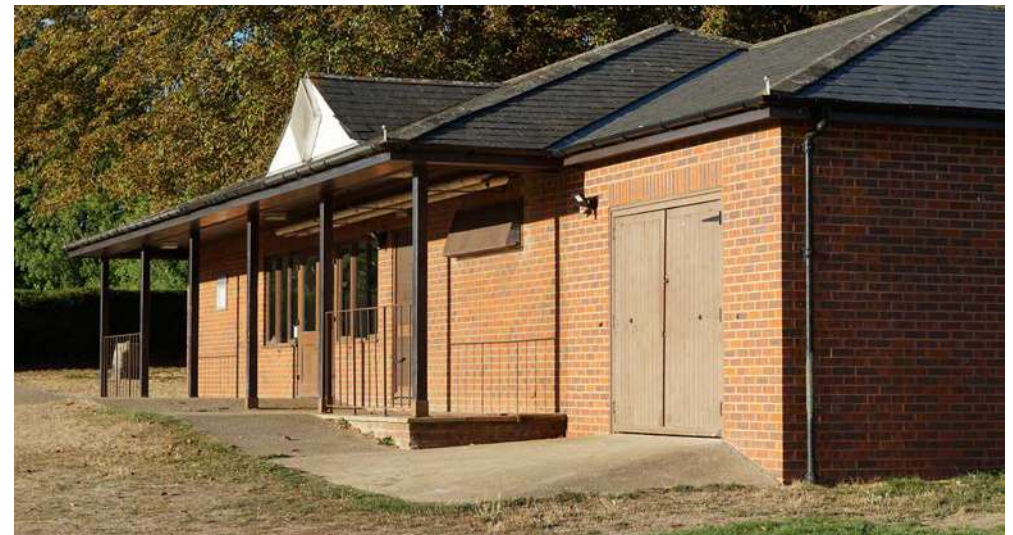
G12.2 - poor appearance of pavilion
